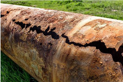
Figure 11: The state of a corroding pipeline (Siraj, 2021)
